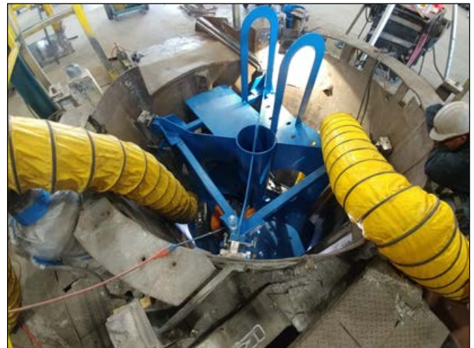
Figure 4. Installers working on the first level jig platform and the new guide rails secured in place ready for welding.
