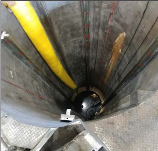
Figure 5. Guide rails and new platen installed as the pit is being prepared for painting.
